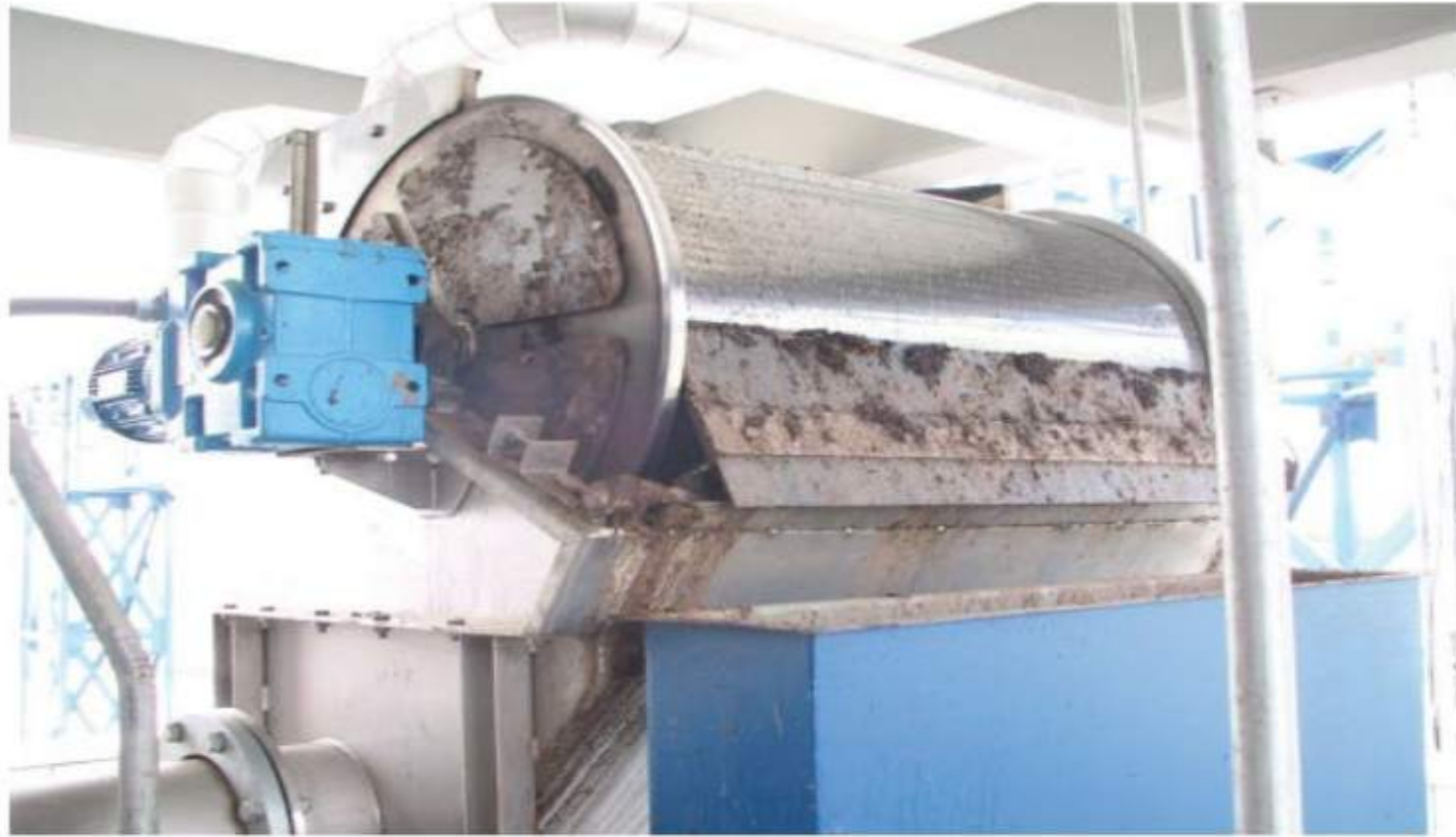
Rotating Drum Screen in operation
