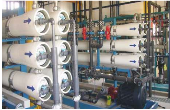
ENTEK Elektrik Üretim A.Ş. (Power Plant) Water Treatment Plant
