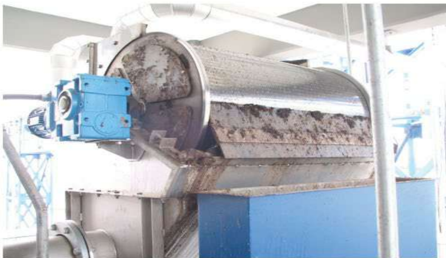
Rotating Drum Screen in operation
