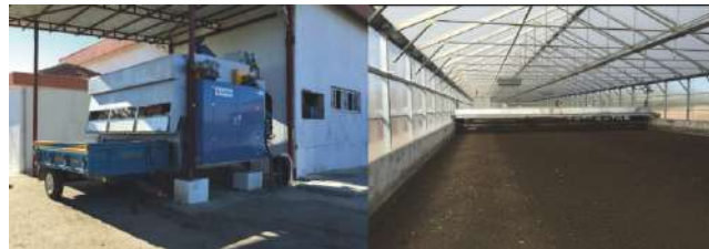
Antalya OIZ WWTP- Construction Year:2015- Capacity: 40 ton/day – 1 pc Dehydrator + 1 pc Solar Dryer Hall
